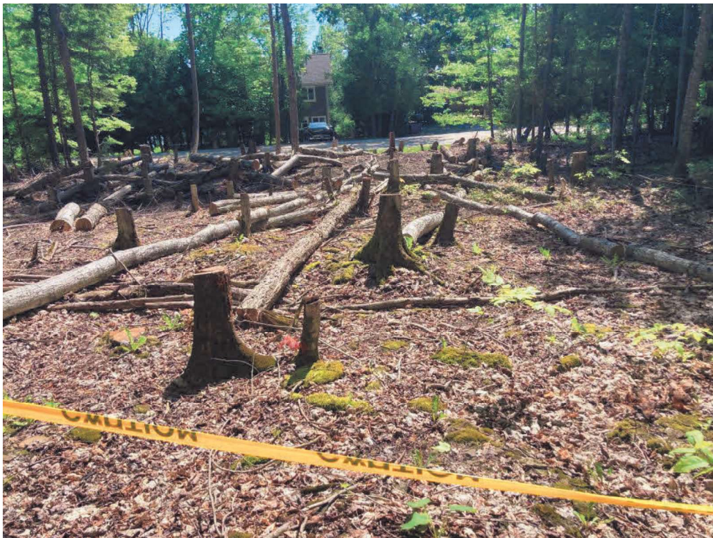
Photo No. 4: Tree clearing area looking east out to County Rd, Note flagging tape perimeter, May 2024
