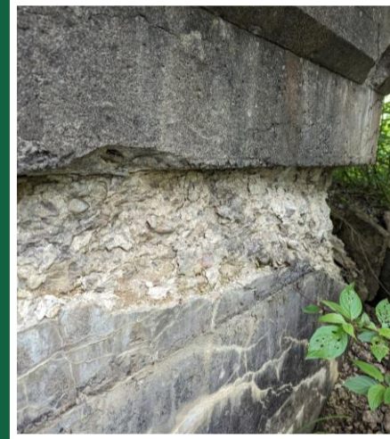
View of Wingwall Deterioration
