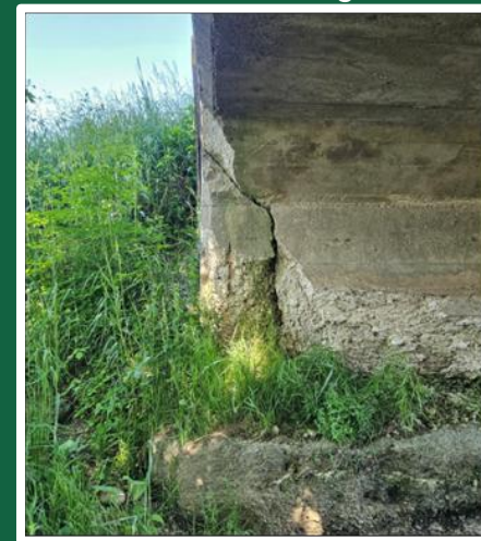
View of Wide Cracking at Abutment/Wingwall
