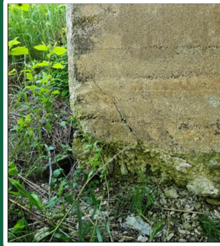
View of Spalling on East Abutment
