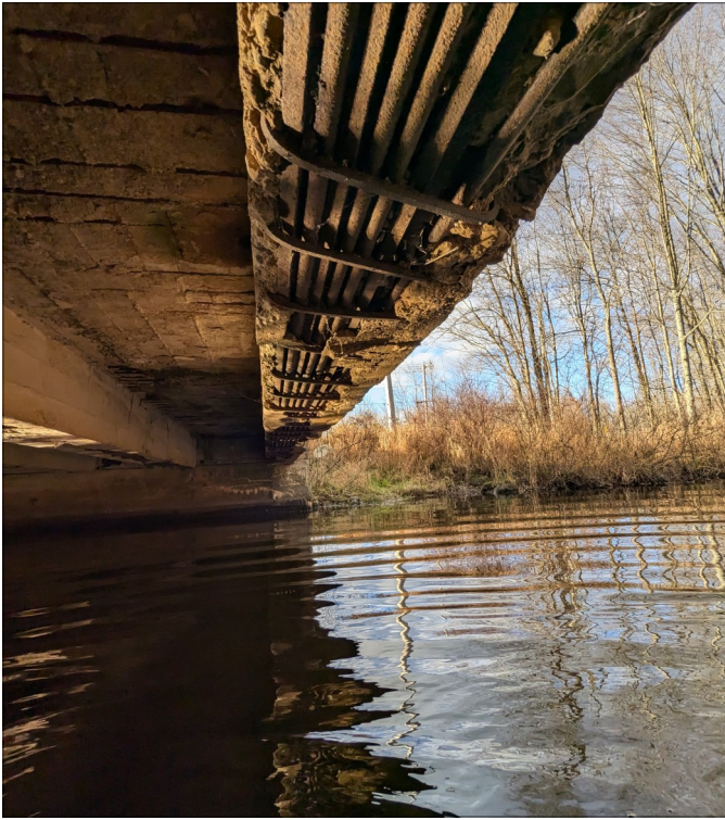
Photo 5 - View of Concrete Structure Girder Deterioration.
