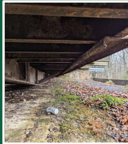
View of Superstructure Corrosion
