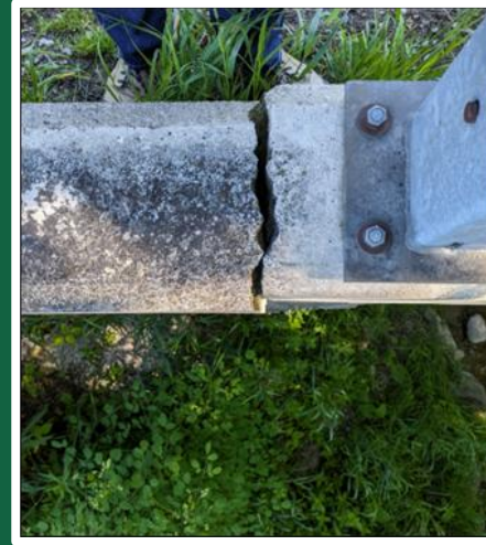
View of Wide Crack & Rotation at Wingwall
