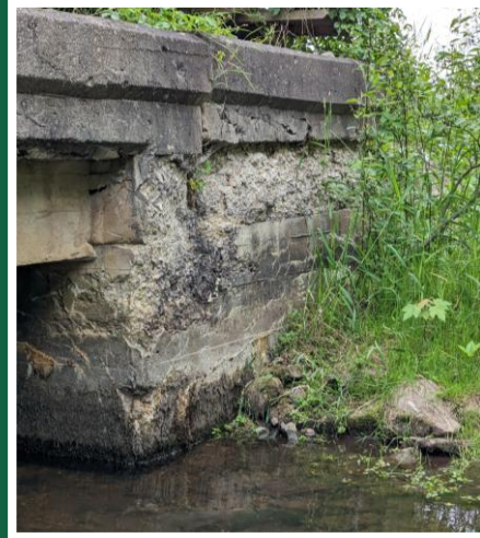
View of Deteriorated Abutment/wingwall
